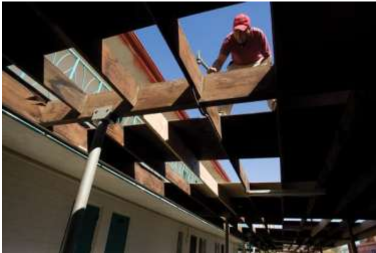
Raymond Solorsano-Agras frames a carport at Shorewood apartments in Phoenix. The Mid-Century Modern property is being renovated by Pathfinder Partners LLC of San Diego.
