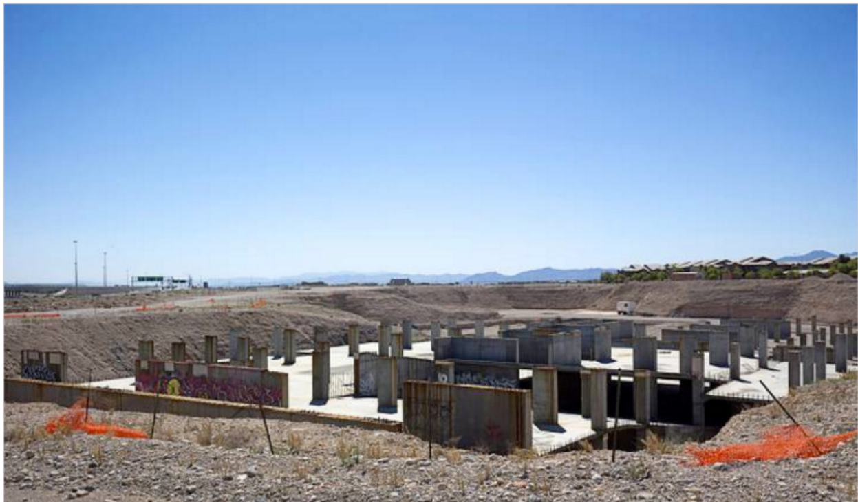
A view of the former Spanish View Tower development site on West Maule Avenue, near Durango Drive and I-215, is shown Thursday, June 16, 2016.
